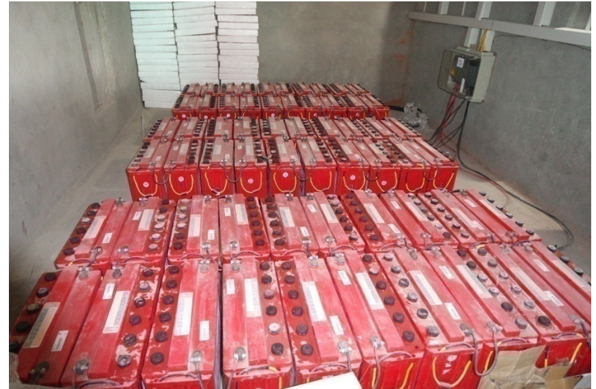
72 batteries of 10000 AH/2V
