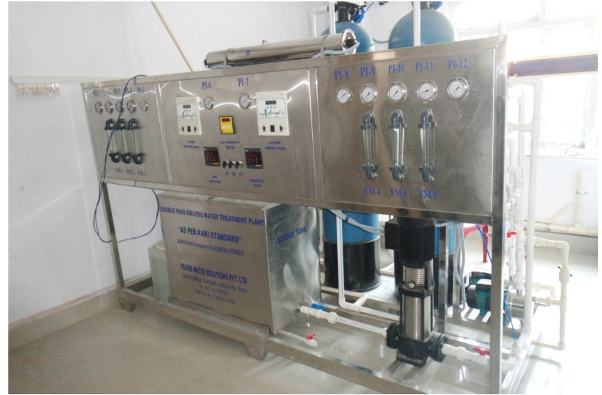
Reverse Osmosis system
