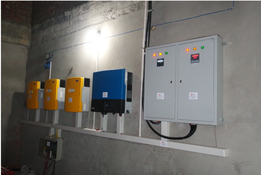
Charge controllers and Inverters
