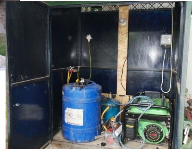
Future target: production of electricity from Bio-gas
