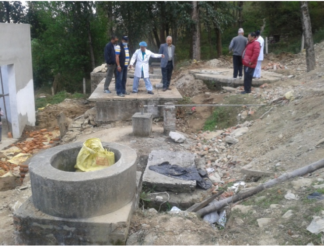
Inlet: food, pathological waste & toilet drainage
